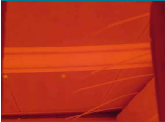
Fig. 10 Bottom of the main Deltabeam after 180 minutes of standard fire.
